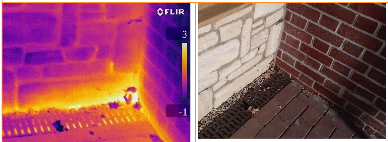
6.46: Thermographic image when building pressurised, showing substantial heat loss at end of ground floor wall, adjacent to pillar
