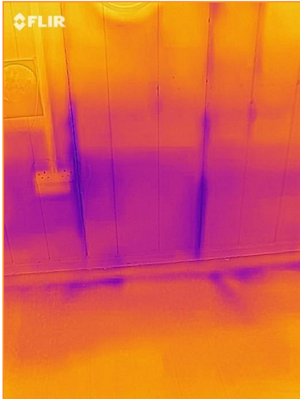
6.34: Internal thermographic image whilst building depressurised, showing heat loss between boards along (1) base of side wall to main hall and (2) along the bottom edge of the skirting board
