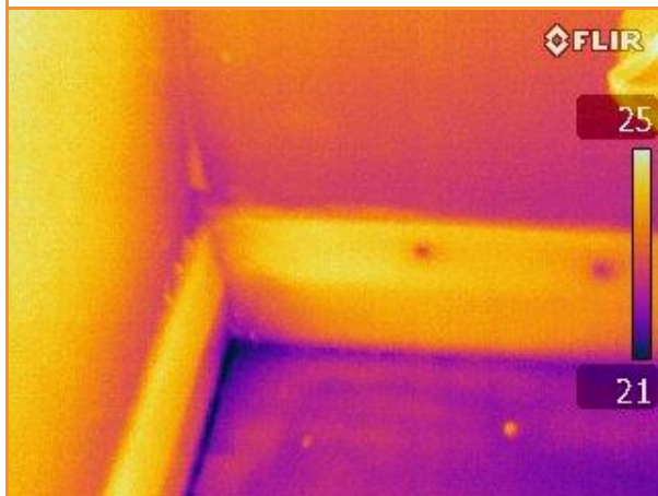
6.30: Thermographic image showing leakage in corner beneath junction of skirting
