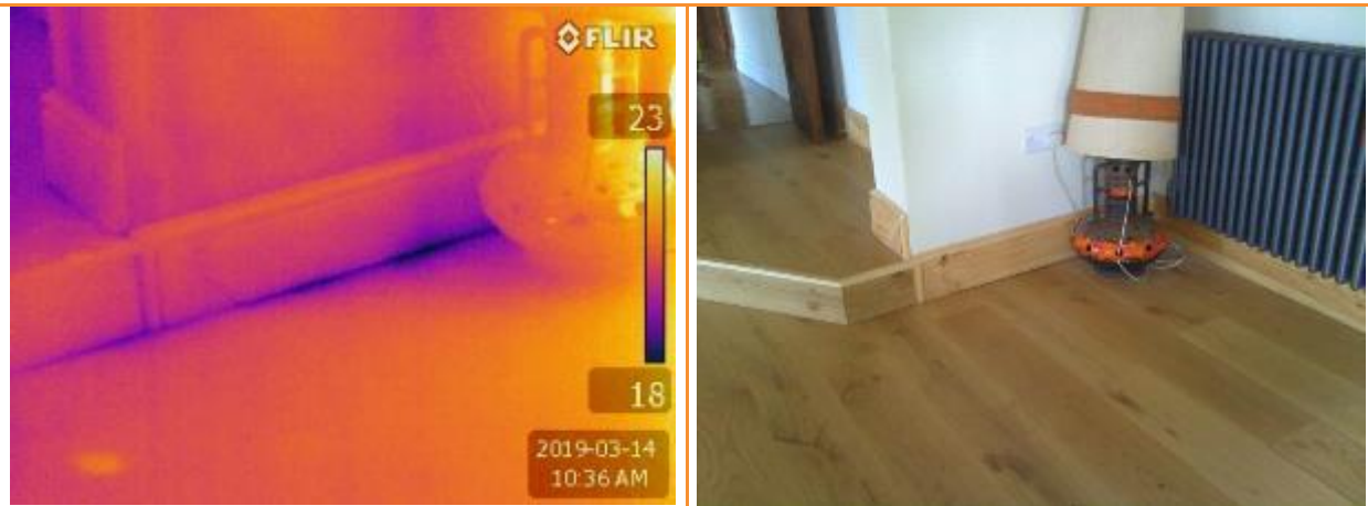
6.02: Internal thermographic image whilst house is depressurised showing leakage along bottom edge of skirting board along internal partition wall.
